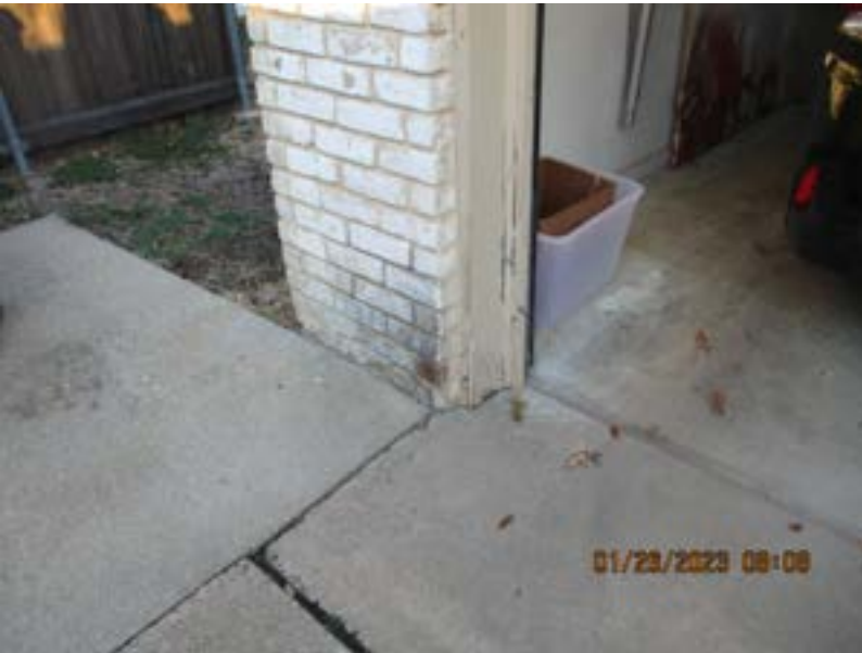
Conducive - Wood Rot (M)
