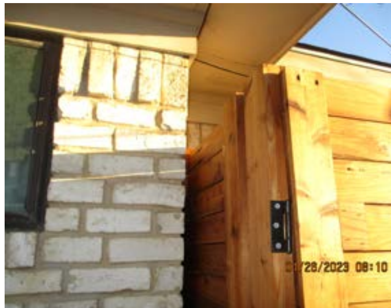
Conducive - Wooden Fence in Contact with the Structure (R)
