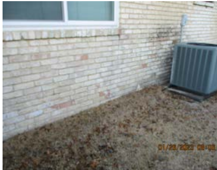
Conductive - Footing too low or soil line too high (L)
